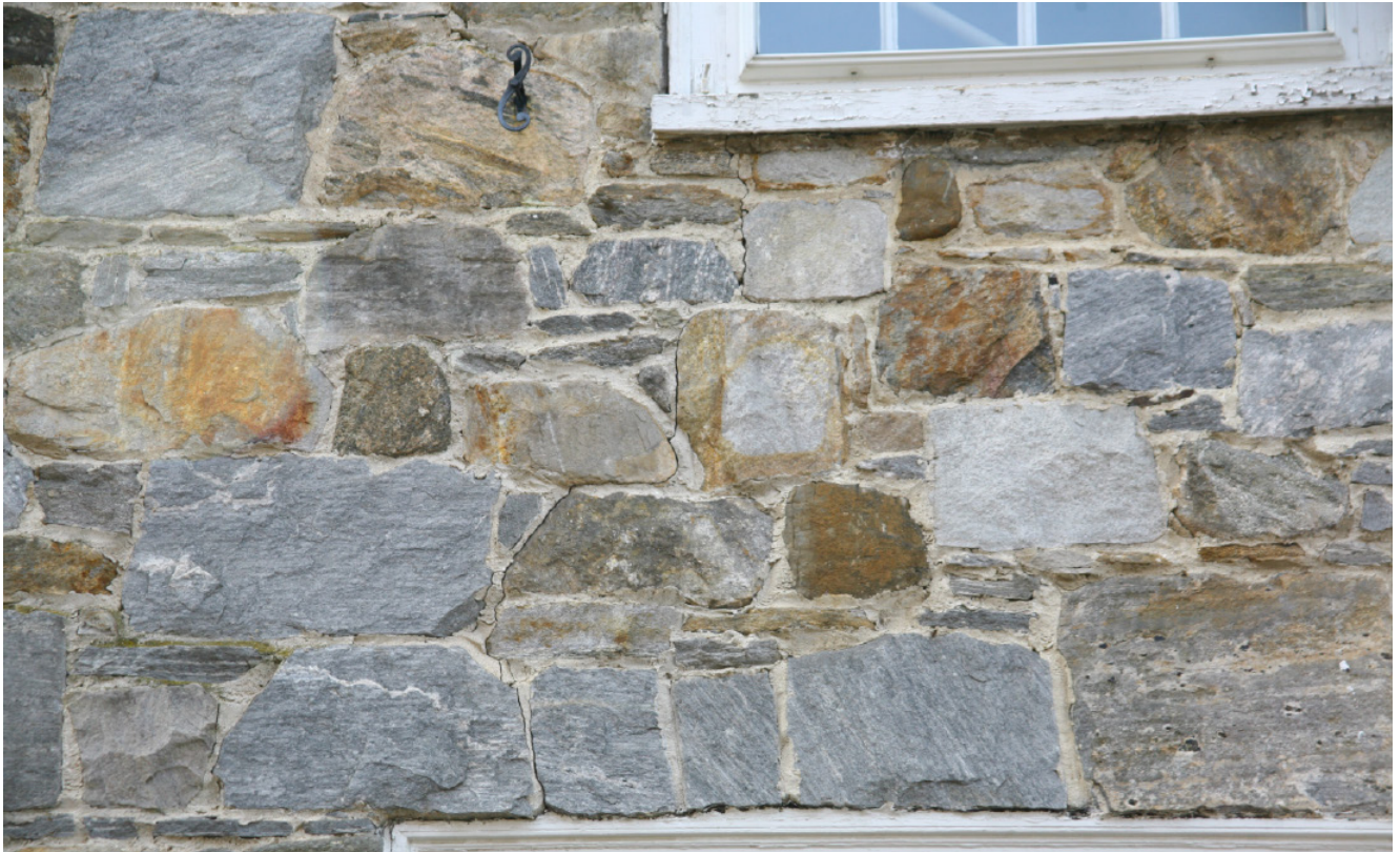
Fig. 37. This is a continuation of the crack seen in fig. 36.
