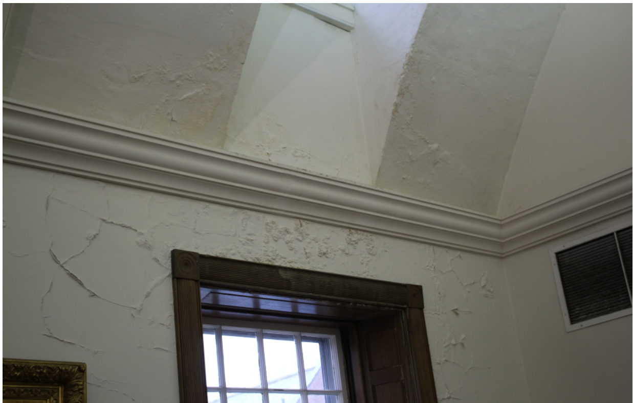
Fig. 53 Southeast corner of the former auditorium. Past water infiltration has caused the gypsum plaster finish to bubble and deteriorate. This in turn has caused the paint finish to fail as well. This is representative of the plaster surrounding many of the dormers and is likely the result of roofing issues.
