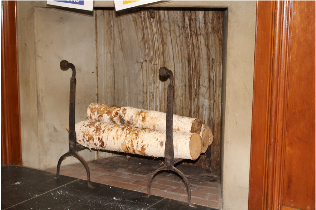
Fig. 54 West wing, second-floor fireplace. Note the water stains in the firebox and at the rear of the hearth. The white debris on the hearth extension is paint and plaster dust from the ceiling above. This location should be monitored to determine the status of water infiltration. The chimney here should be capped if it is not already.
