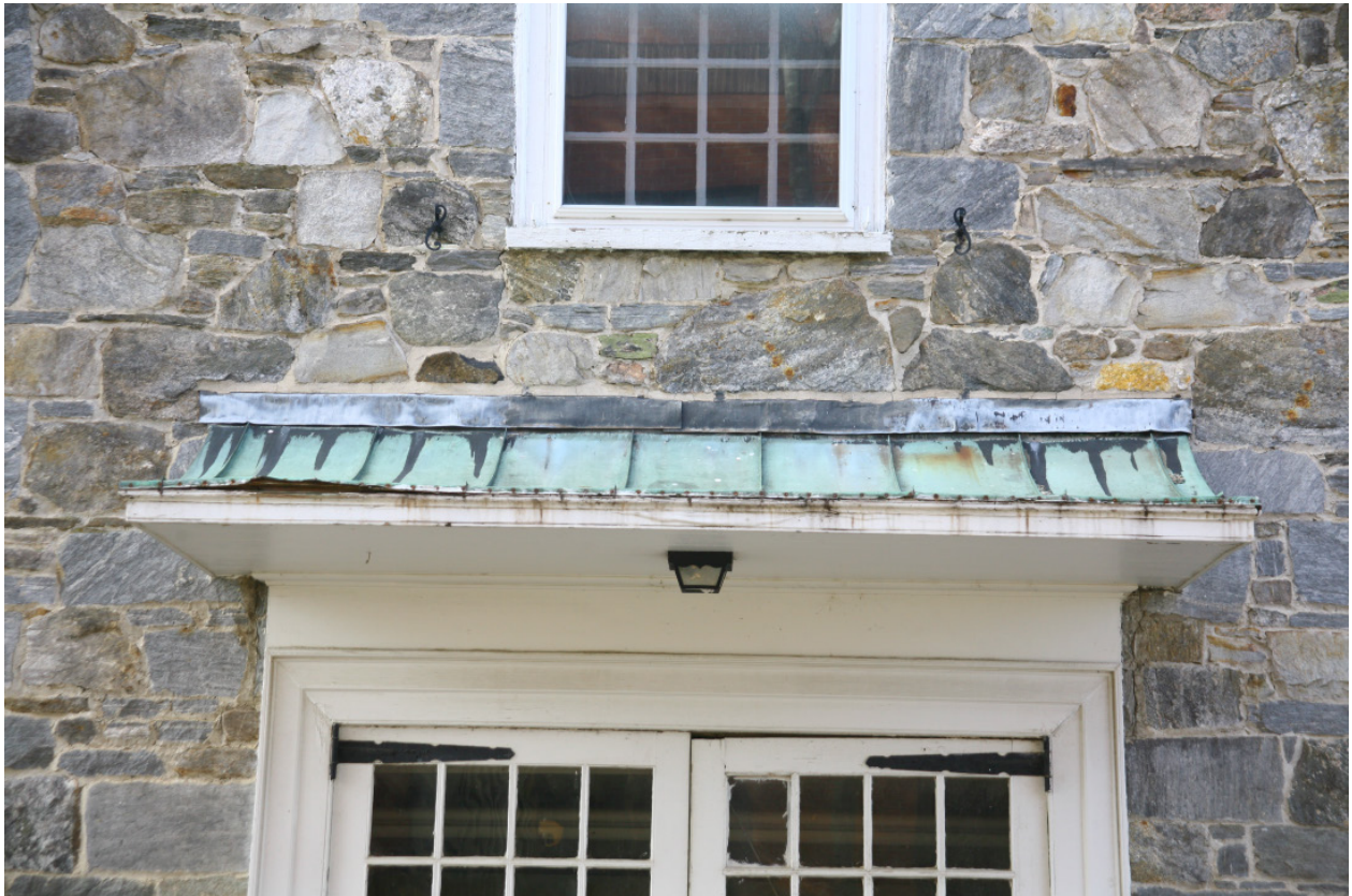
Fig. 31 Copper roof at east barn doors. The roof is lifting away at the left end and is generally in poor condition. It has served its purpose and is at the end of its useful life. This roof should be replaced in-kind with new standing-seam copper roofing.
