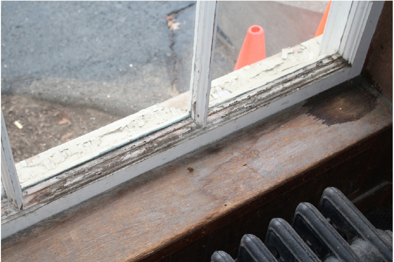
Fig. 45 Representative examples of failing paint on the window sash and water-stained sills. These conditions are typically the product of condensation that forms on the window glazing and eventually drips down onto the sash and sills. The sill also looks to be dried out due to failure of its clear coat and decades of UV exposure.
