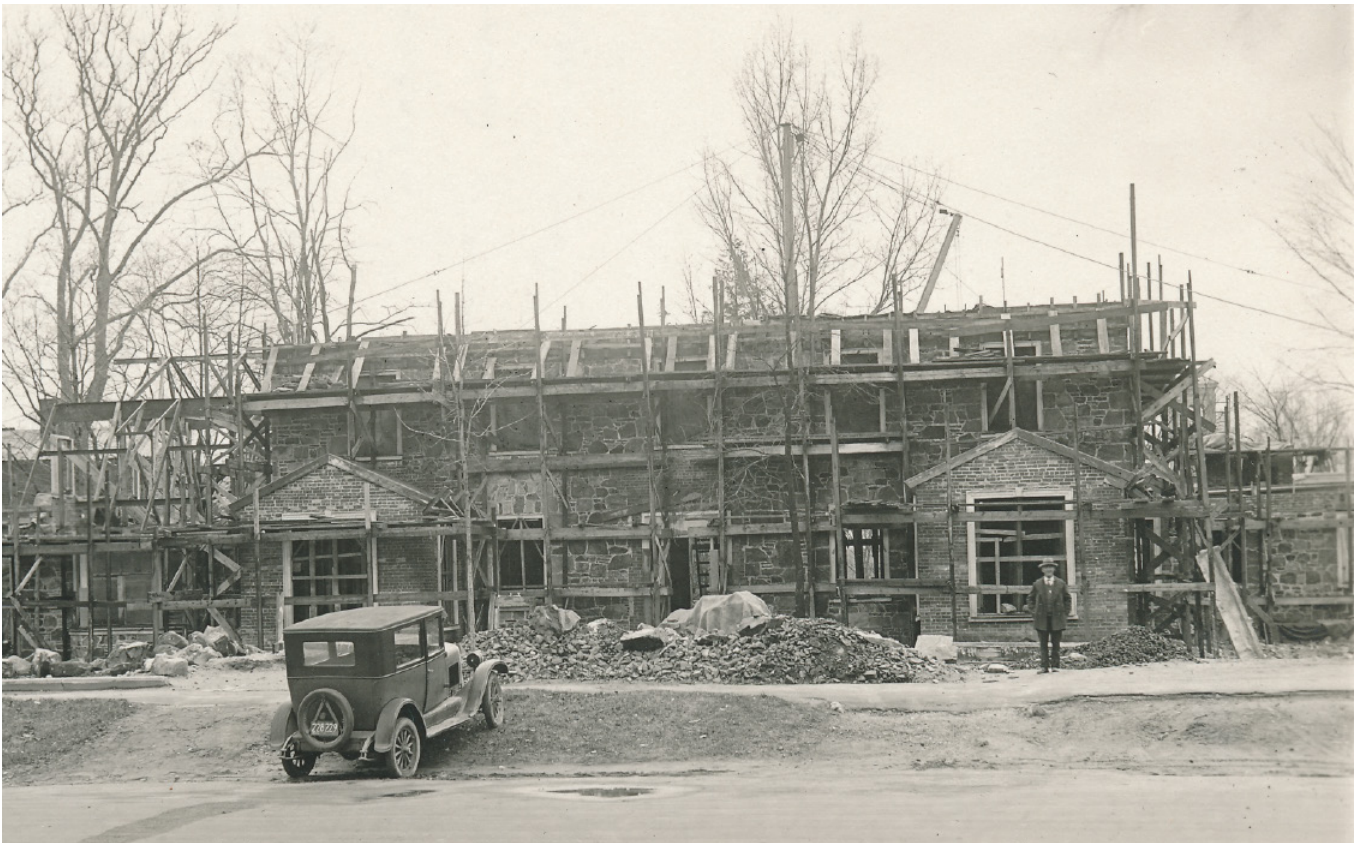
Fig. 40 Jones Library under construction. The sun porches are brick and steel like the rest of the building's construction. The steel roof frame can be seen on the west wing at the left of the image.
