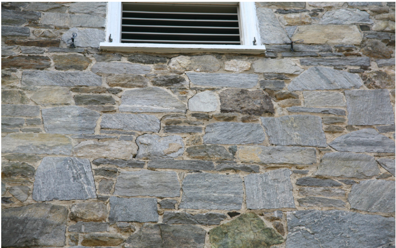
Fig. 36. East elevation of the east wing at the north end. Note the vertical crack running up the center of the image.
