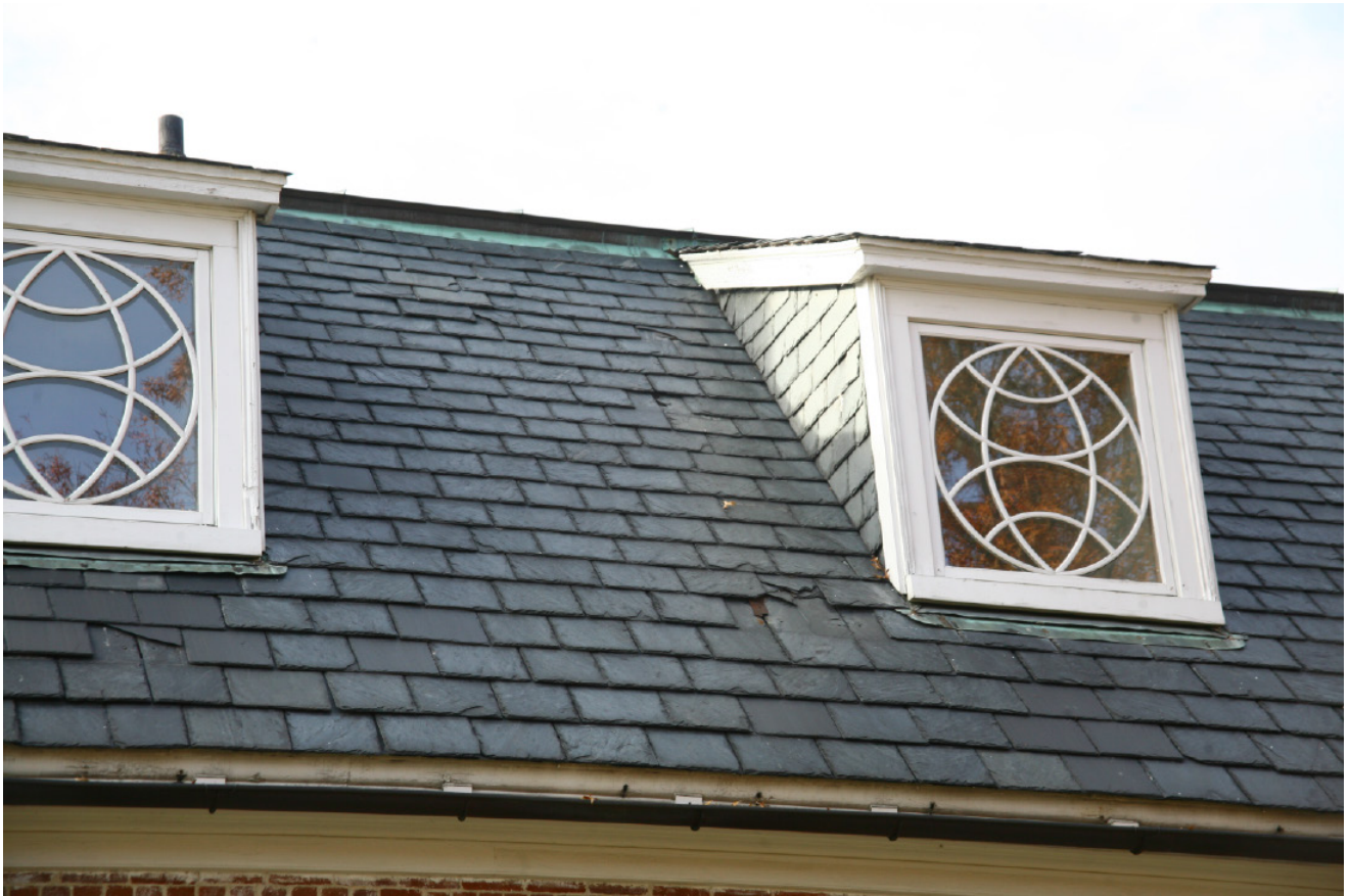
Fig. 29 Detail of slate roof, east wing. Multiple missing and broken slates. The conditions here are representative of what is seen elsewhere across the roof.
