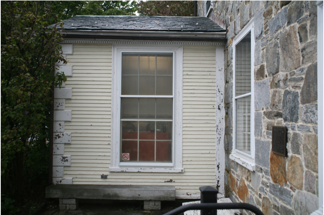
Fig. 41 West sun porch, east elevation. Like much of the woodwork on the building, the paint on the sun porches is in poor condition. All of the painted surfaces need to be prepped and refinished with a high-quality paint system that includes priming areas of bare wood along with two top coats of finish paint.
