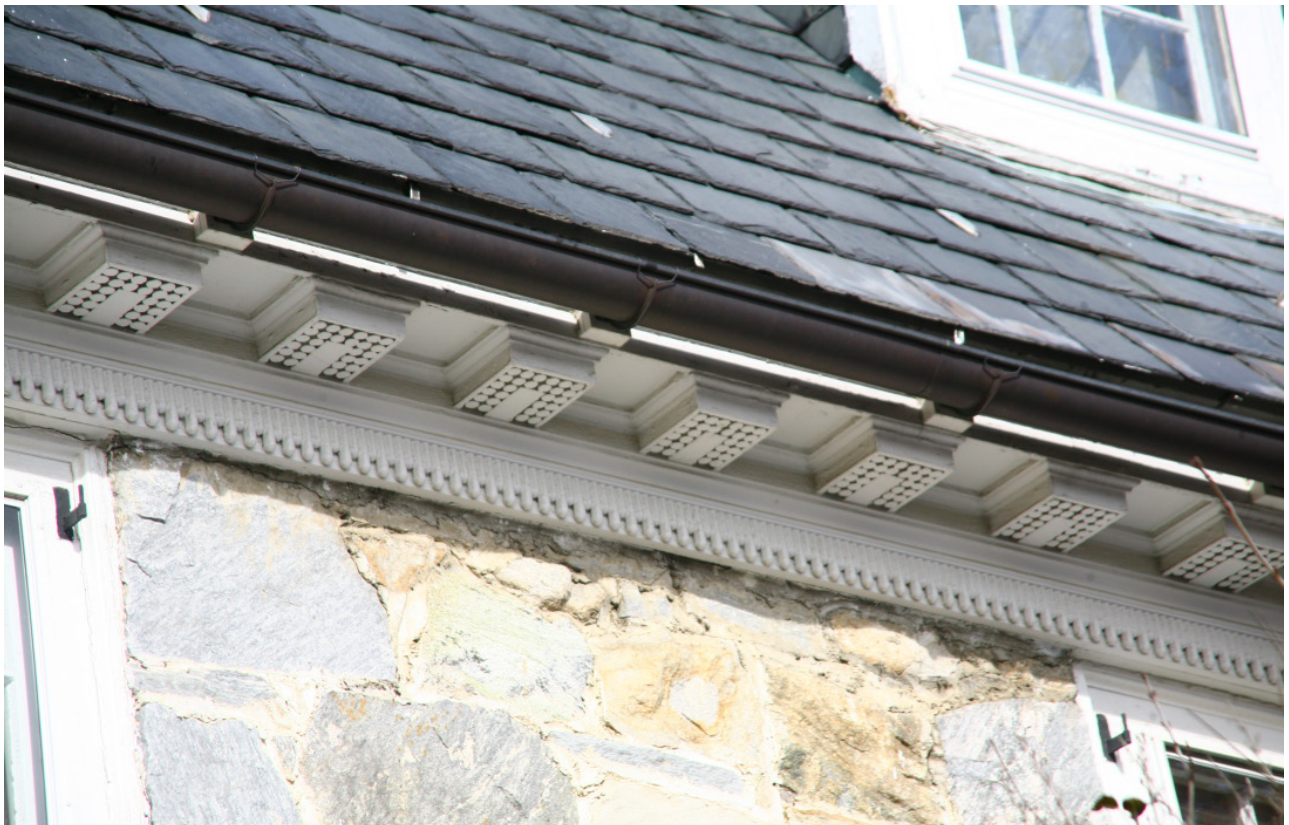
Fig. 34 Detail of the decorative wood cornice found on the building. Note the half-round copper gutter in front of the cornice and shutter hardware at the window openings.
