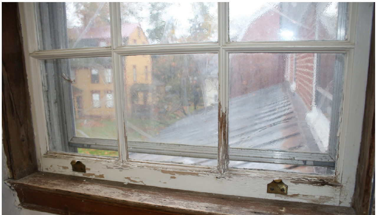
Fig. 46 West wing, second-floor north window. This window exhibits the typical failures seen from condensation and UV damage. The window is situated in what appears to be a problematic location, where the upper roof discharges rain and snow onto the lower roof (seen through the window). Being the north side of the building, it likely holds moisture and snow longer than elevations that receive direct sunlight.
