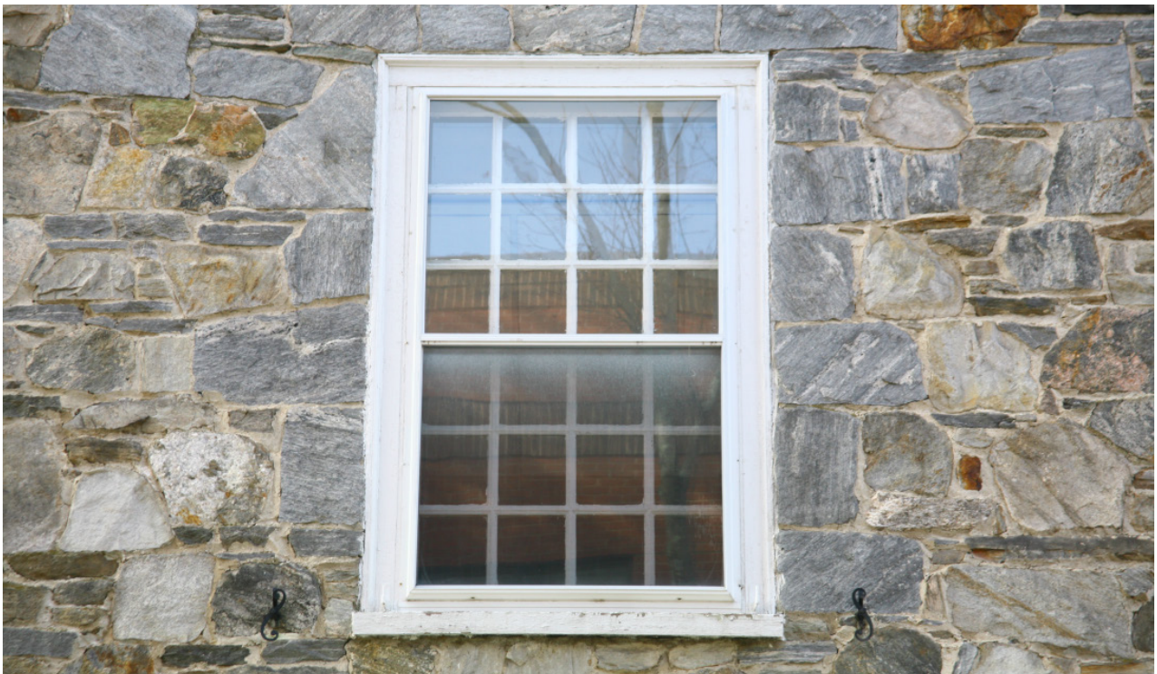
Fig. 42 Typical 12-over-12 divided-light wood window found in the building. The wood windows are character-defining features of the building and should be repaired and retained throughout. The existing storm windows are at the end of their service life and should be replaced with high-quality, low-profile storm windows. Notice the holdbacks mounted in the masonry on either side of the window for the shutters.
