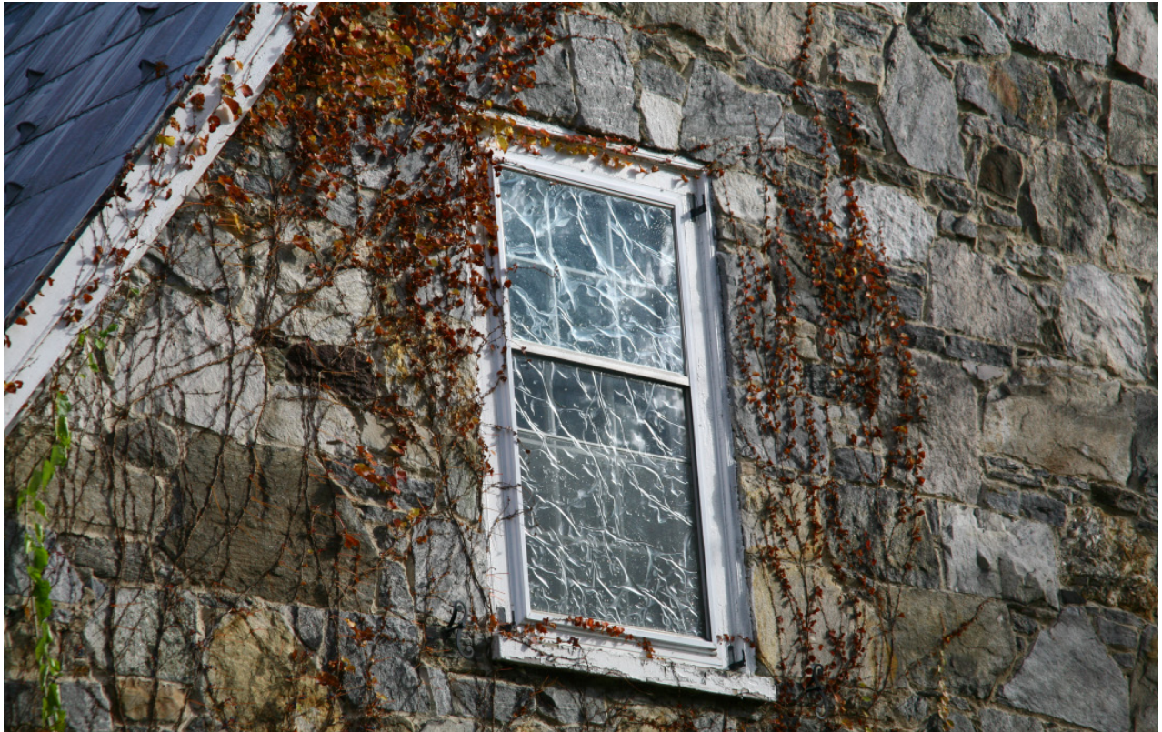
Fig. 44 Many of the storm windows on the third floor of the library have had UV-protective film applied to them. The film is well past its service life and is now bubbling and peeling from the surface of the glazing. Owing to the age and quality of the storm windows, it makes the most sense to replace them with a high-quality, low-profile storm windows.
