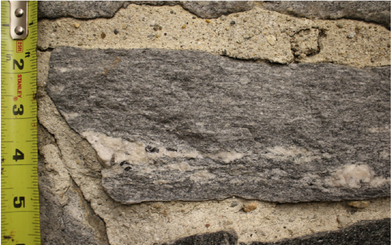
Fig. 35 Detail of mortar in east wall of Special Collections. This closeup shows the color and texture of the original pointing mortar used in the building. This mortar is much different in appearance than that used to repoint the chimneys. Notice the variety of aggregate in the sand used. Any replacement mortar should be formulated to match the color of the original mortar and applied to match the profile and texture as well.
