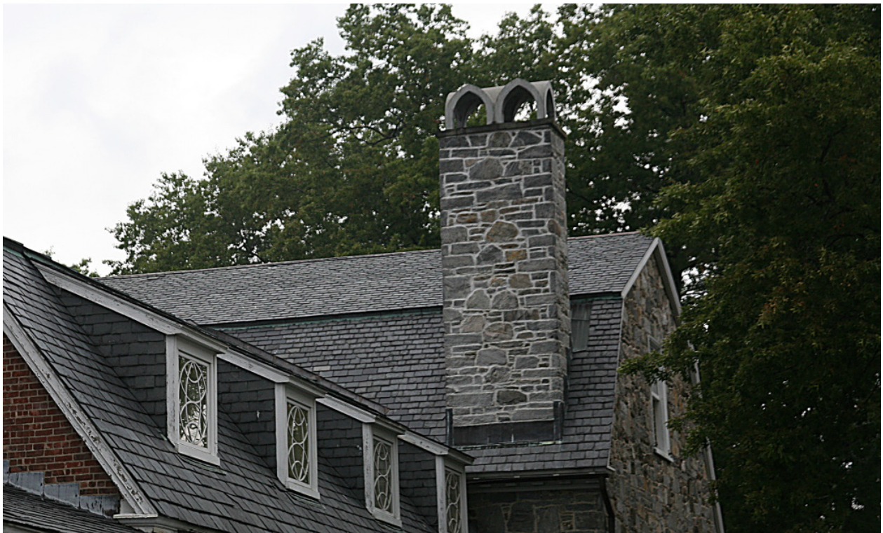
Fig. 32 The modern mortar used to repoint the chimneys lacks the variety of color and texture found in the original mortar. Given its uniform gray appearance, even set high up on the building it stands out.
