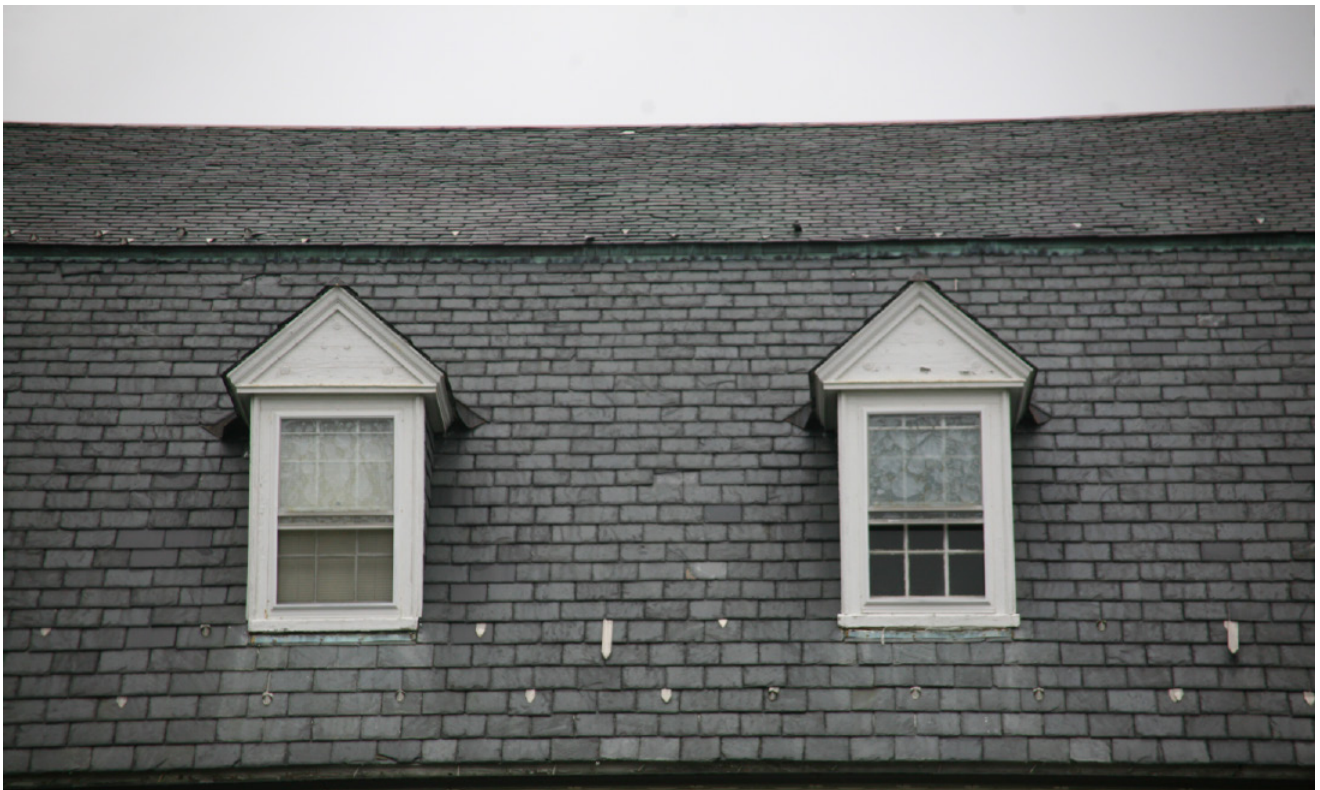
Fig. 30 The slate roof was laid with a graduated exposure, so the lower slates show more of their surface to the weather than those nearer the curb (where the pitch of the roof changes). Notice the snow guards that have slipped and the random broken slates.
